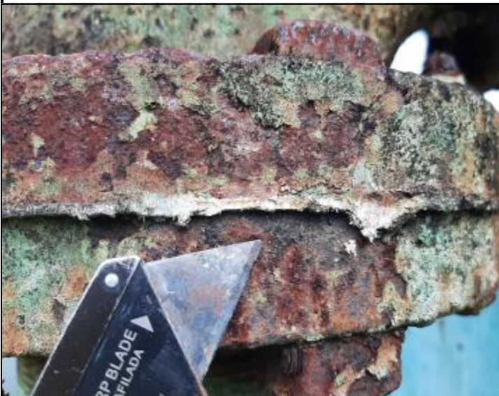
Photographs 02-04: Pipe Gasket; Sample ID 182014-A01, 02, A03
